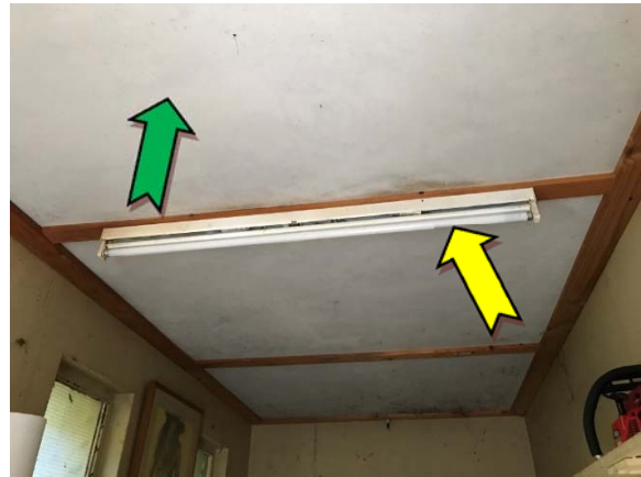
Photo 4. Interior, store, ceiling and single tubed fluorescent light fitting – non asbestos-containing fibre cement sheeting and suspected PCB-containing capacitor.
