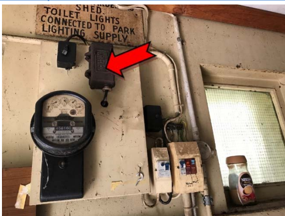
Photo 5. Interior, store, fuse – suspected asbestos-containing millboard insulation.
