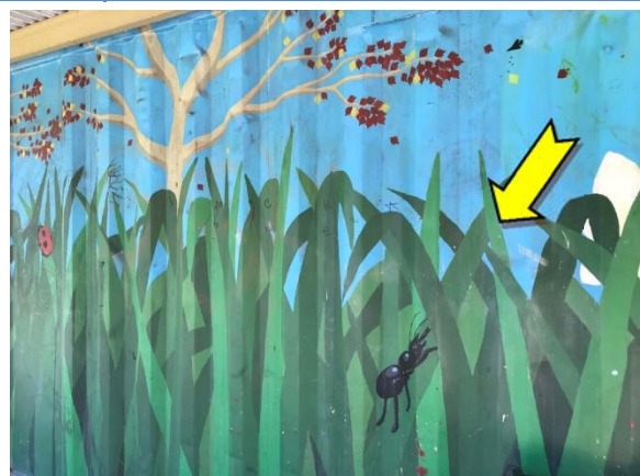
Photo 6. Exterior, graffiti wall – suspected lead-containing various upper coloured paint systems.
