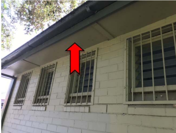
Photo 1. Exterior, throughout, eaves – asbestos-containing fibre cement sheeting.
